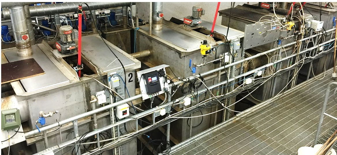
Figure 4. Photo of the top of biological treatment tanks BR2-4
